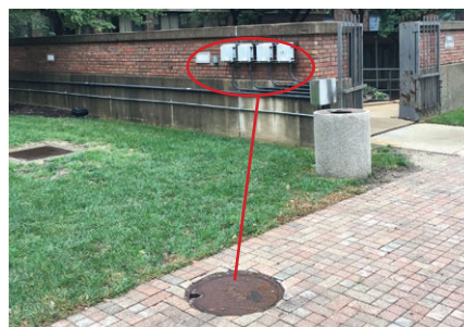
Unit can be mounted externally (remote monitoring)
